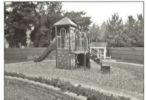
After - new play structure with landscape design, garden beds, and play house.
